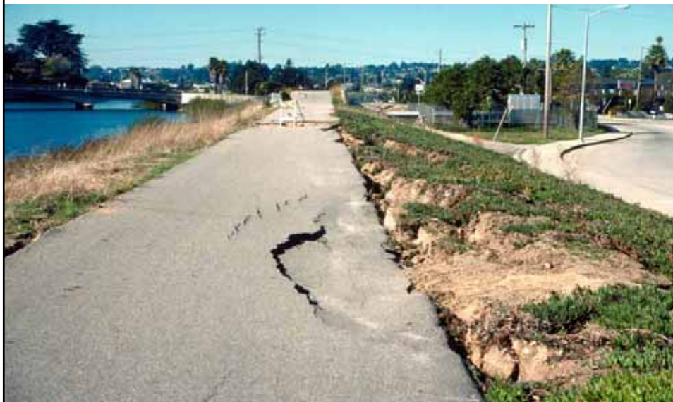
1989 Loma Prieta Earthquake damage to San Lorenzo River Levees (10/1989)
