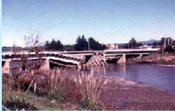
Soquel Ave Bridge after Jan. 4-5, 1982 flood
